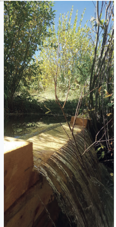
Completed simulated beaver structure along Fall River with water spilling over from the pond.
